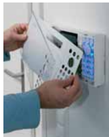
Easy panel and keypad installation
